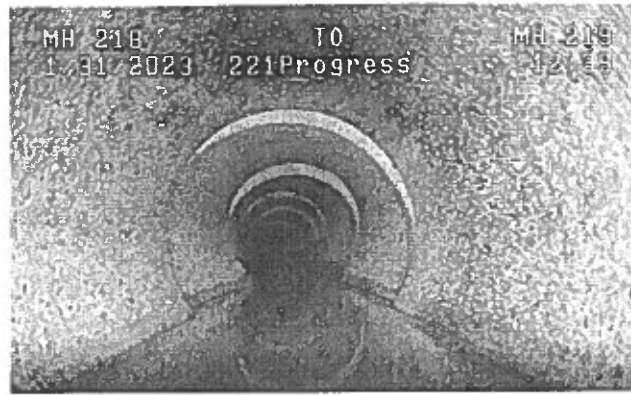
Figure 2: Progress Street – Joint Separation(119.6')
