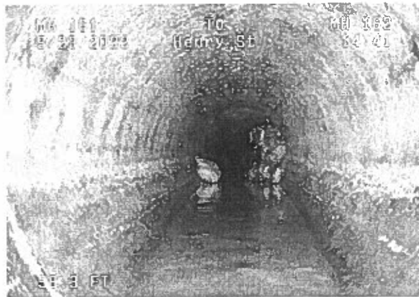
Figure 4: Henry Street – Tree Roots
