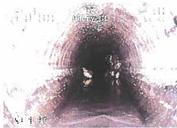
Figure 4: Henry Street – Tree Roots
